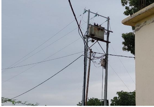
Figure 3: MV/LV power line to be reinforced
